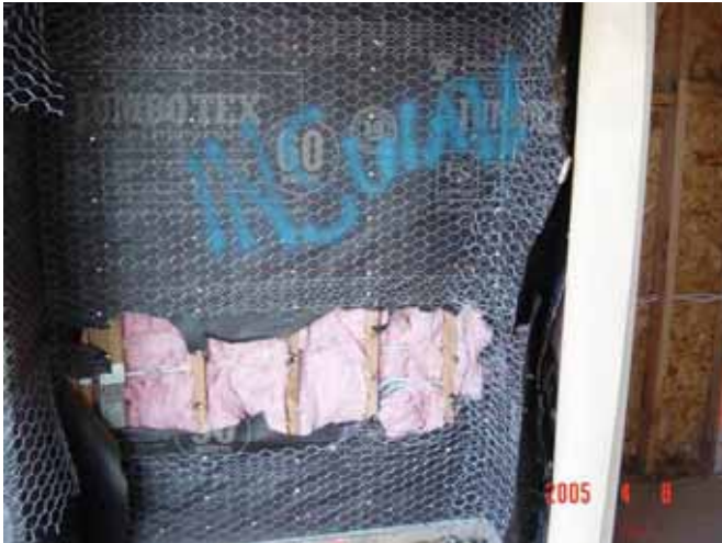
Figure 3. Electrician had to run last minute wiring, builder insulated lower portion at this time.
