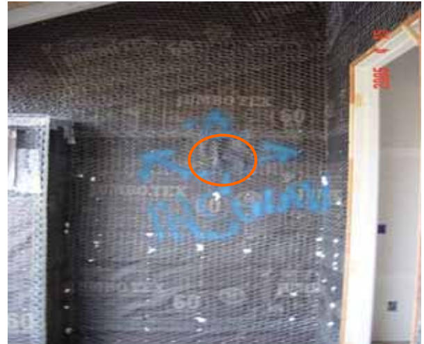
Figure 4. After hole cut in top portion of wall to show missing insulation (figure 2), builder patched hole over.
