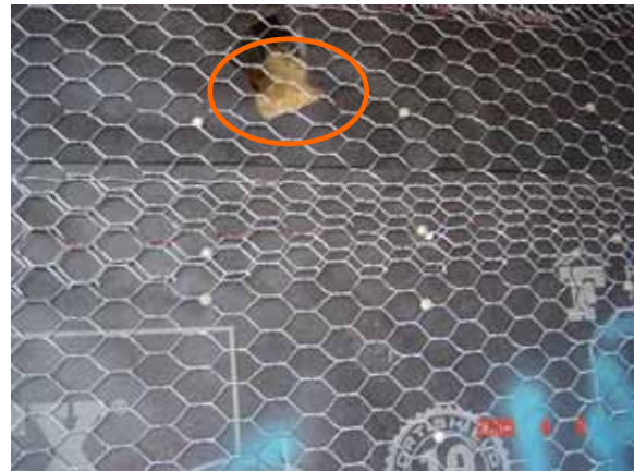
Figure 2. A small hole was cut in exterior paper confirming suspicion of missing insulation.
